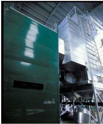
CoopeDota's new, state of the art burners
